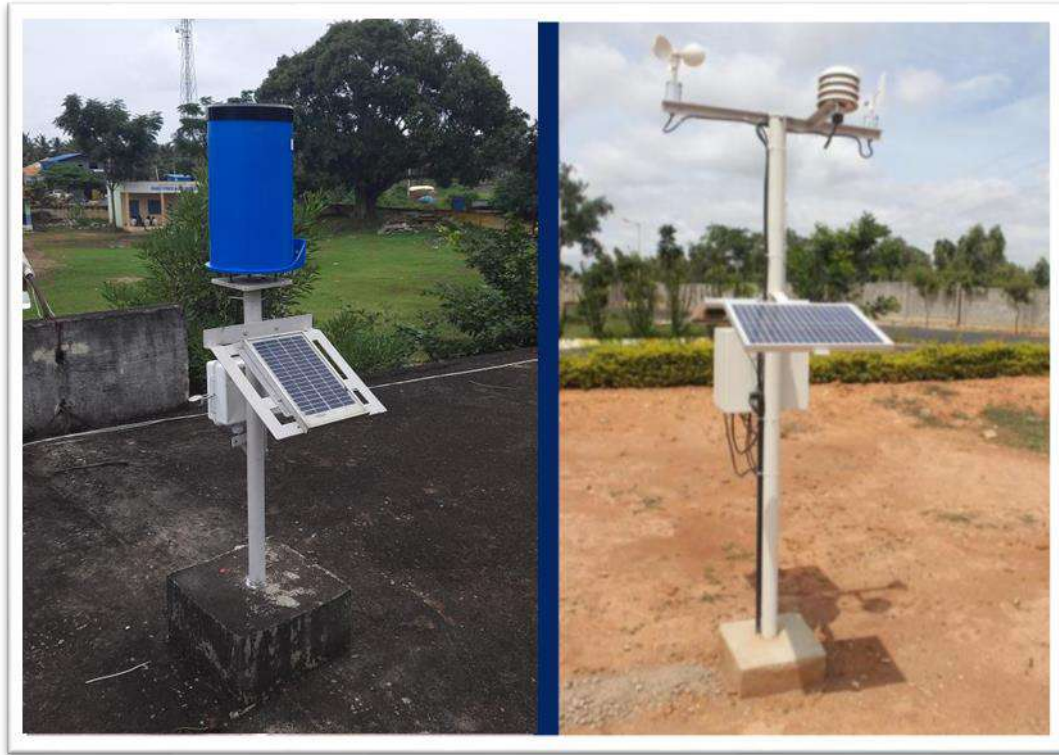
Telemetric Rain gauge
