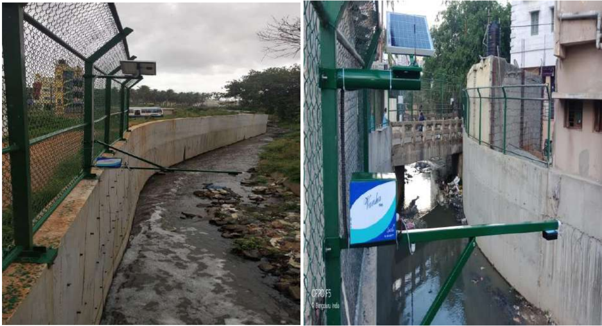
Figure 9: Water Level Sensors at Doddabidarakallu & Doddabidarakallu
